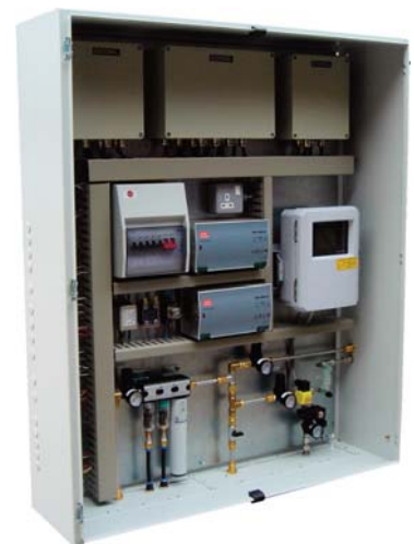
GCEM4000 CEMS Control Panel
